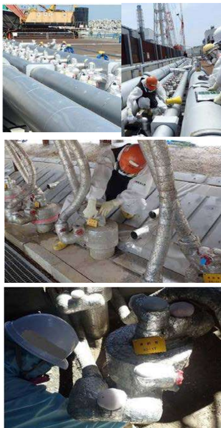
Figure 5: Planche photos de la mise en route de la congélation (Source Tokyo Electric Power Company Holdings, Inc. Date June 6, 2016).
